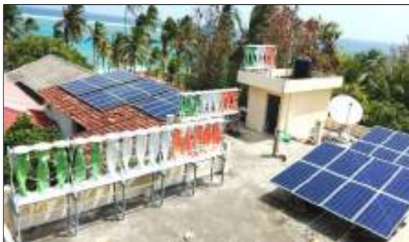
Powering Ice Plant at Lakshadweep
